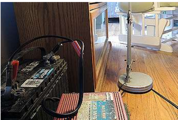
Car batteries at the Doroski house power some lights.
