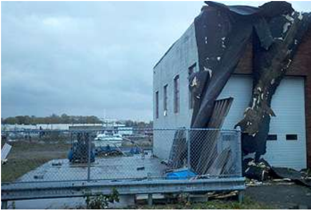
The roof of the mainenance shop at the Ocean Church marina was torn off by 80 mph winds.
